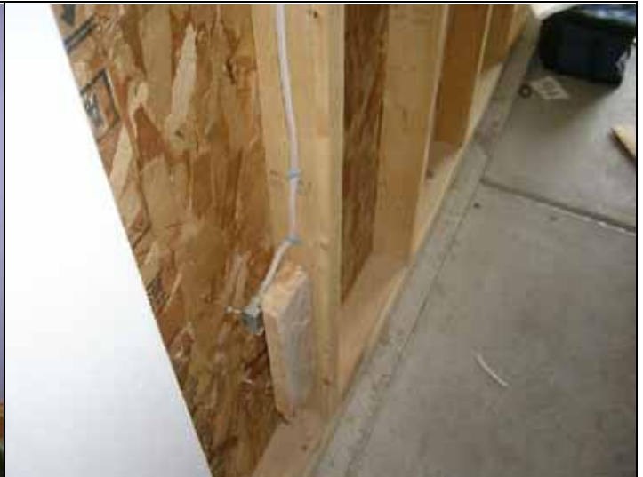
Exposed wiring in garage
