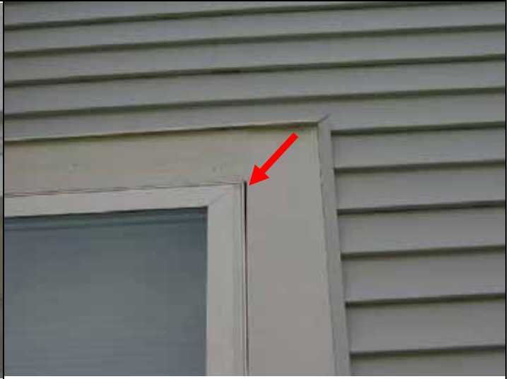
Caulk around windows
