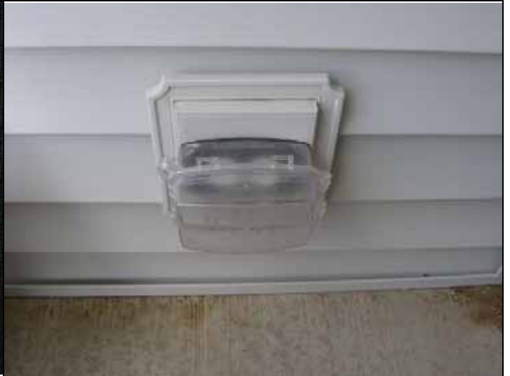
Loose outlet in entrance area
