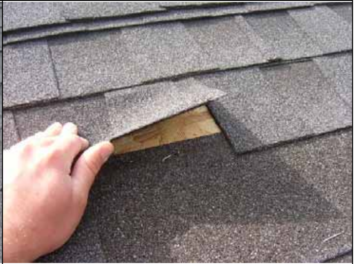
Leakage can occur, no underlayment
