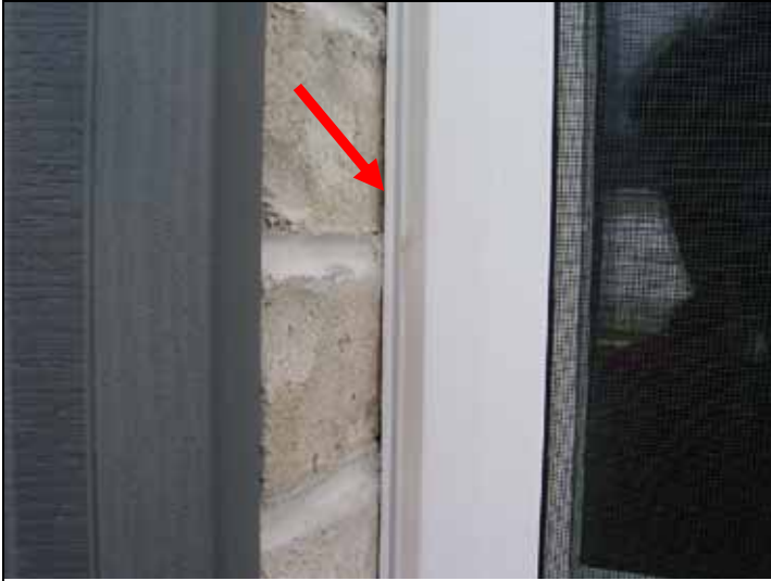
Caulk around windows
