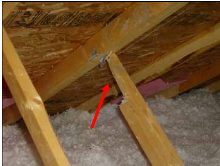
Truss cord was damaged and will need to be replaced.
