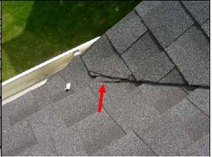
Loose shingles, sloppy cuts
