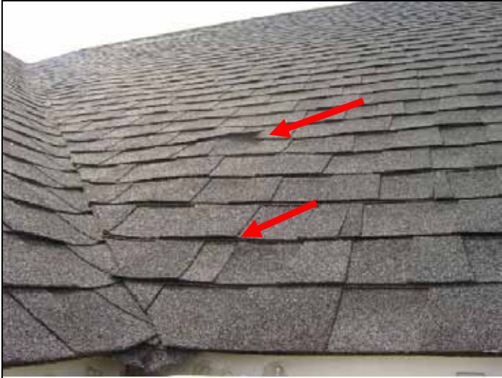
Several shingles not sealed, staples popped
