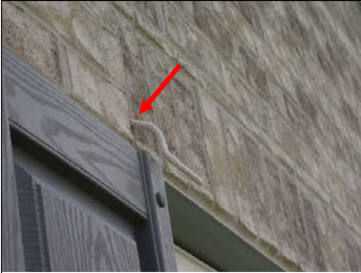
Ropes need trimming
